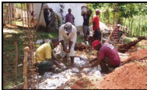
Haitian workers prepare the foundation for the Guest House sponsored by Sylvania Franciscan Health.
